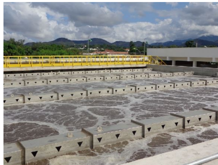
Figura 31: ETE Deodoro (Vistoria DIS/GFT)
